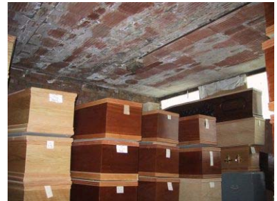
The storage area had constant leaks, causing expensive damage to coffins and caskets.
