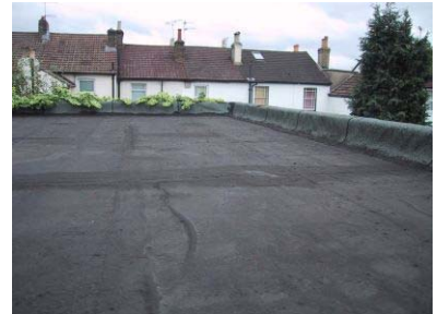
The entire roof was repaired many times (by professionals) but the leaks did not stop!
