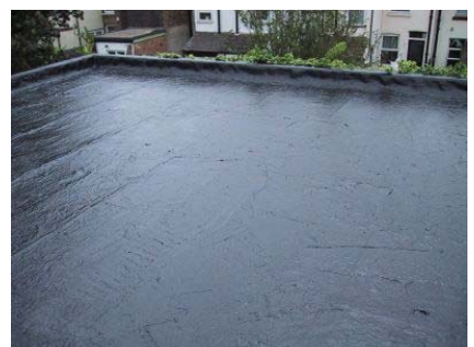
The roof was entirely waterproofed/finished within 2 hours, providing protection that can last more than 10 years.
