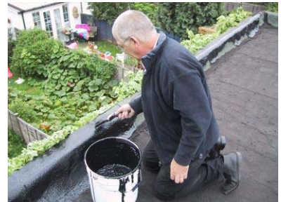
Shakespeare's do a spot of DIY, and find out just how easy it is to apply. One coat of Roofix 20/10 solves all the leaks.
